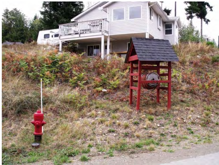
Photo 2 Dashwood Volunteer Fire Department hydrant and strata hose reel, Country Road in Little Qualicum River Estates.
